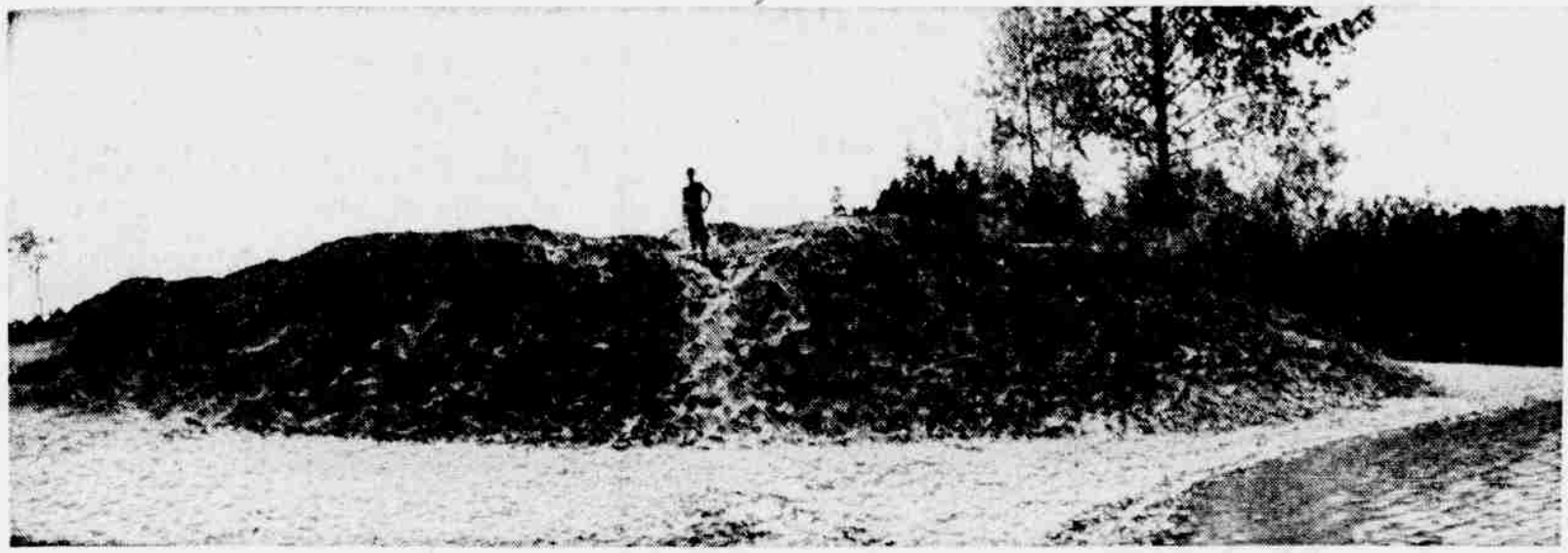
SOON TO BE BEACH this 4,000 cubic yard mound of sand was dropped on the shores of Elk Lake last week to extend Eagle Park Beach on the southeast corner of the lake near Pat Bay
