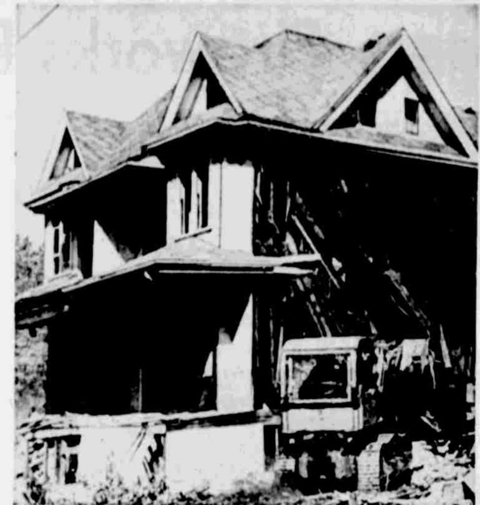
AND THE WALLS CAME TUMBLING down . . . on top and around bulldozer operator Ray Bryce who, after nibbling away at the corners, does a
